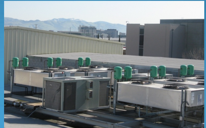
Typical Data Center Installation
